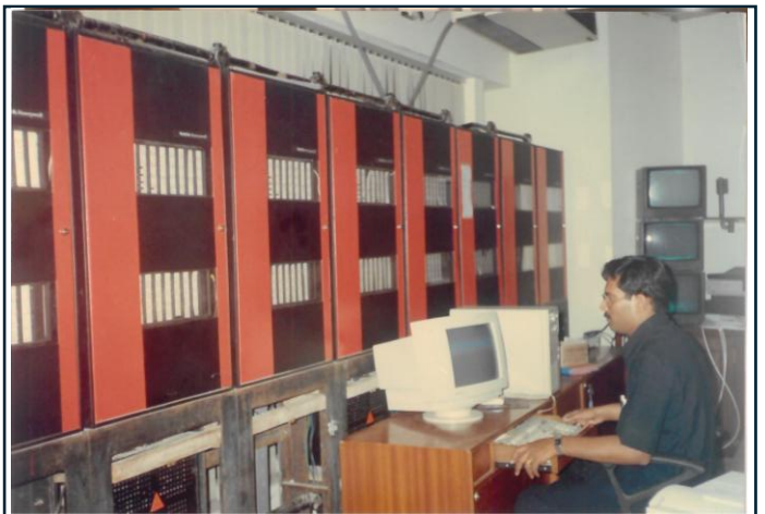
1994 to 1996 Officer – Security & Fire Safety ESSAR HOUSE, BMS Room
